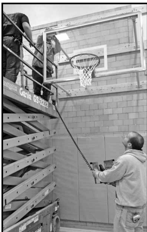
(Photo by Michael Carnes) City recreation director Alex Koch helps position his co-workers so they can finish installation of one of the new basketball hoops at the Wayne City Auditorium.
